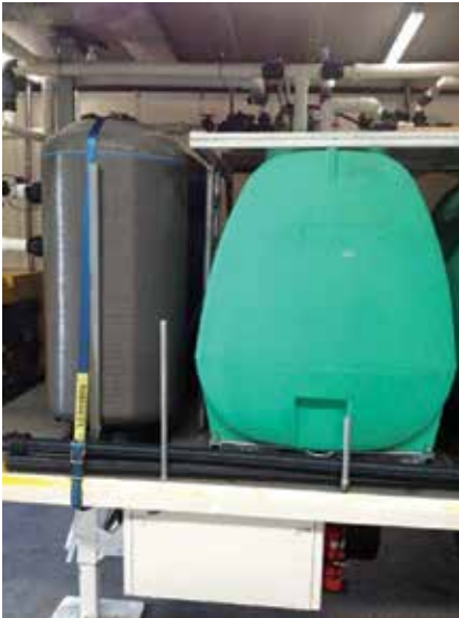
Waterco filters in conjunction with an ion exchange filter media.
