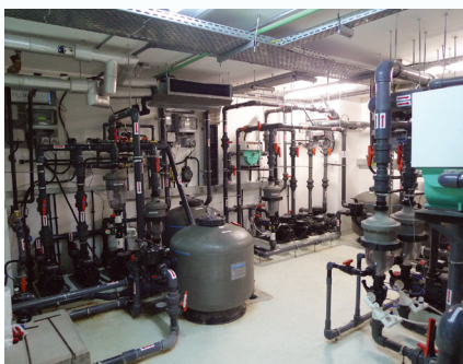
Hydroxypure with inbuilt remote monitoring, 12 Supatuf pumps, six MultiCyclones and five Micron media filters complete with Waterco glass bead media.
